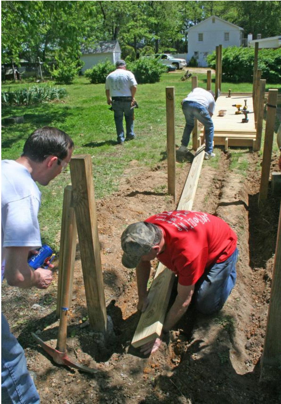
Christmas in April volunteers work to install a new handicapped accessible ramp at a home in Loveville April 27
