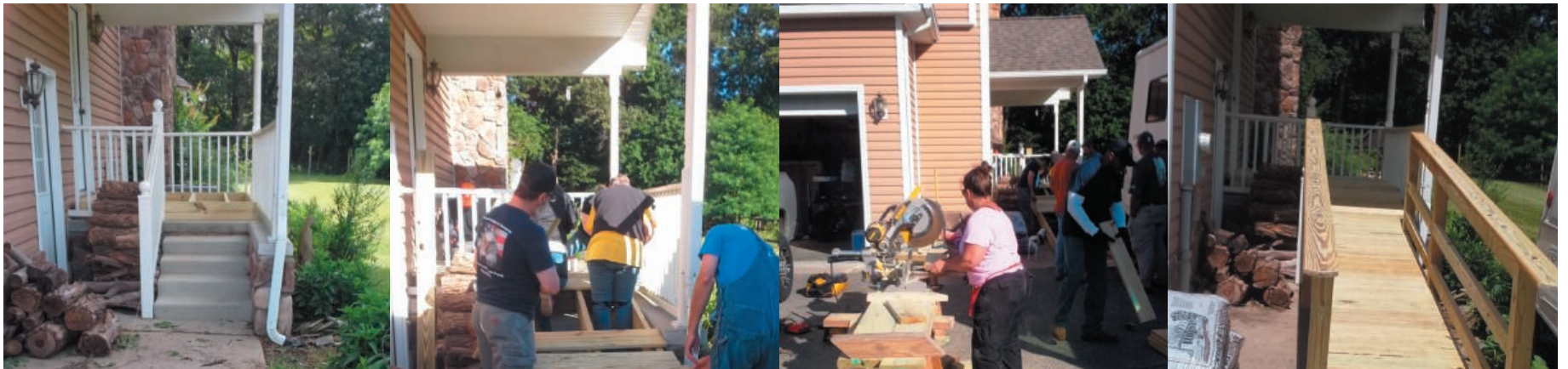
Pictures show work being done on the Smith home by volunteers from Patuxent Habitat for Humanity, Christmas in April, Calvert County, Exelon Militaries Actively Connected (EMAC) and several other organizations.
