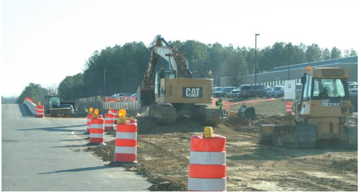
Construction on Airport Road in California makes way for the 3rd Building of the University System of Maryland at Southern Maryland
