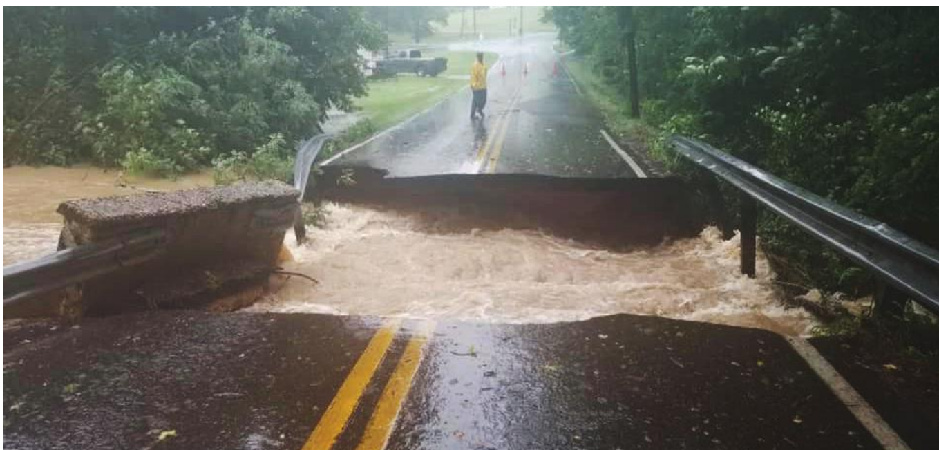
A local road washed out following Isaias
