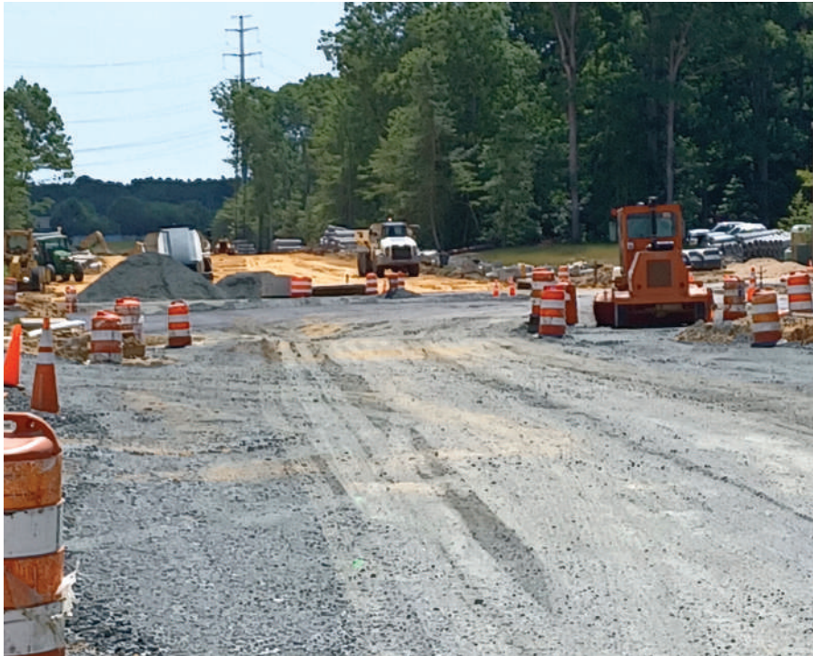
The most recent work on FDR Boulevard at the intersection with Chancellors Run Road
