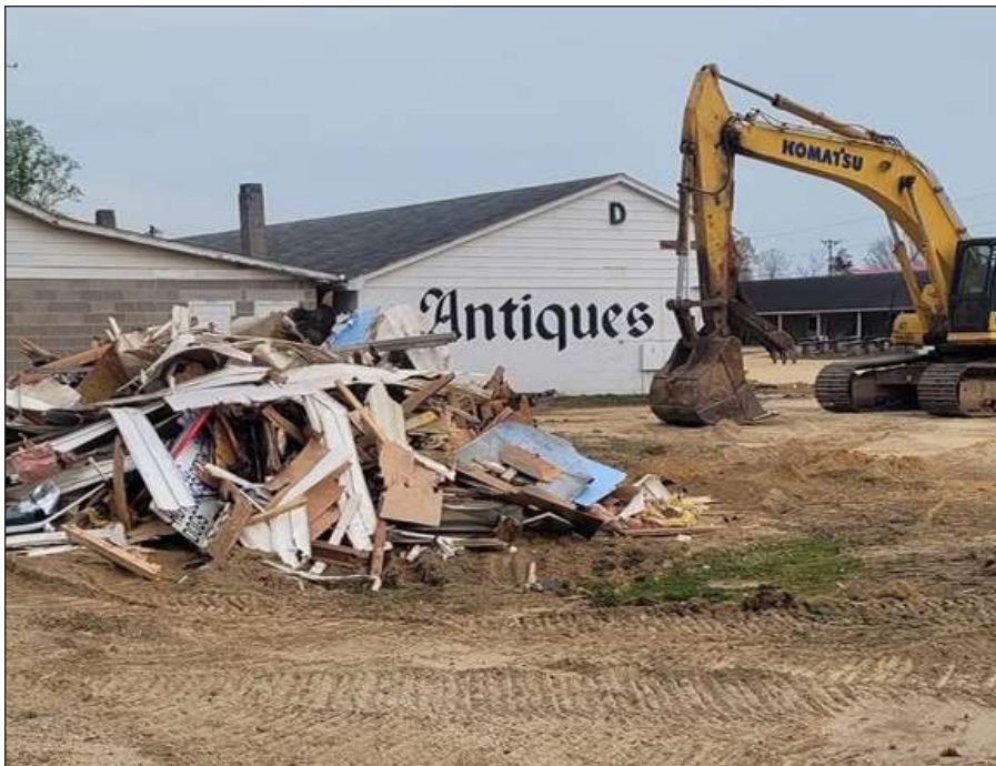
Demolition began last week on the old Charlotte Hall Farmers Market which stood for decades in the northern reaches of St. Mary's County. It drew dozens of vendors of all kinds and thousands of people to shop there each weekend.
