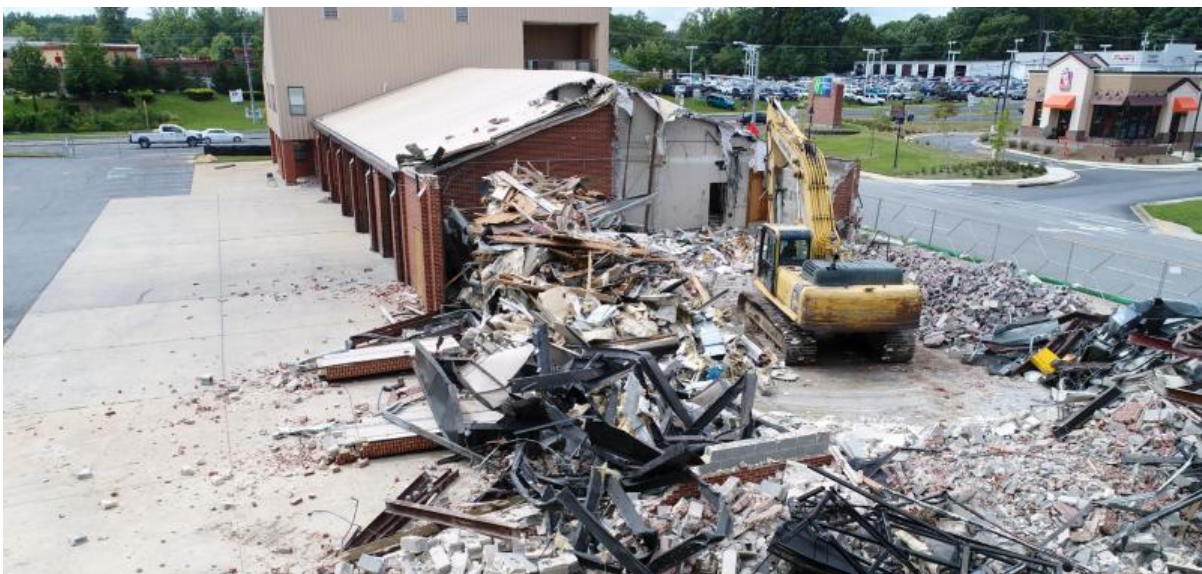
Demolition in late August of the old Prince Frederick Volunteer Fire Department firehouse.
