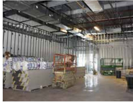
Construction has begun on the College of Southern Maryland's Velocity Center at Indian Head, a 13,400-square-foot facility that will feature a 280-seat multipurpose room, two 24-seat classrooms, two 16-seat seminar rooms, an eight-person executive-style conference room, Makerspace and Flex Office spaces. The facility will open during Spring 2020.
