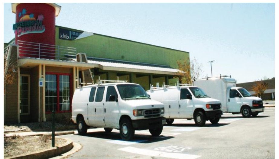
Contractors have been working on refurbishing the vacant Cheeseburger in Paradise restaurant to make way for a Greene Turtle franchise, county development officials said.
